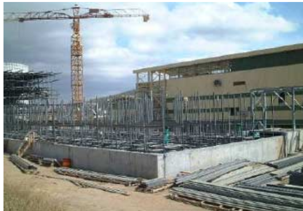
Figure 4 - Olkaria II Project
